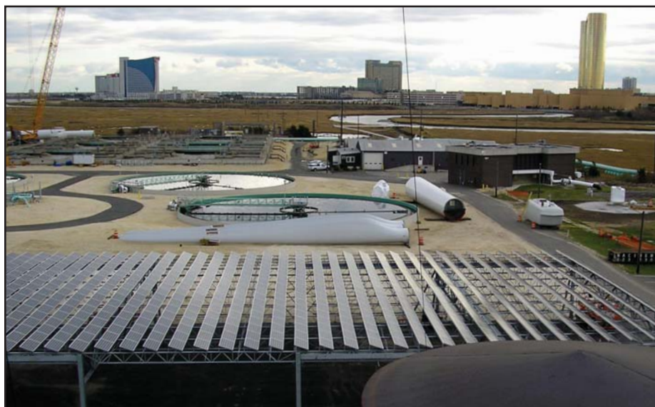
■ Fifty-two rows of PV, each consisting of 18 modules, form a canopy over the carport at the ACUA wastewater treatment plant.
